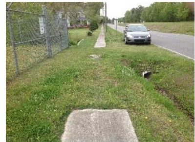
Section of missing sidewalk along North Main Street.
